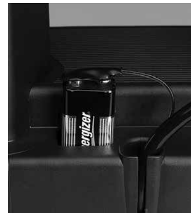
9-V-block battery for the emergency lowering
